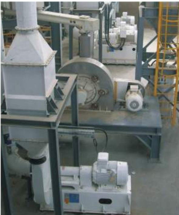
2. SMW 63 in a coating installation with stearic acid melting vessel
